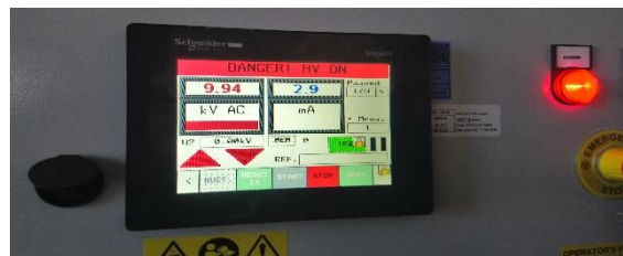
Fig.3a. High voltage sources display (during test)
